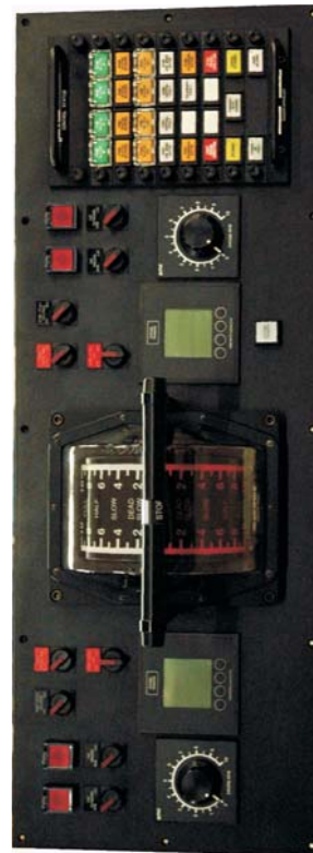
Engine Control Room Plate
