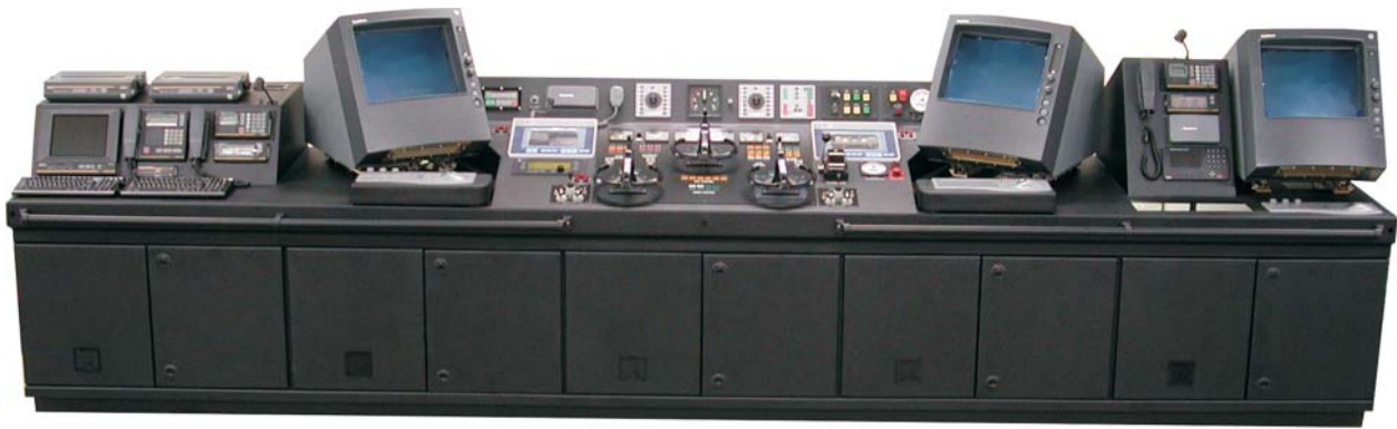
CENTER BRIDGE CONSOLE
