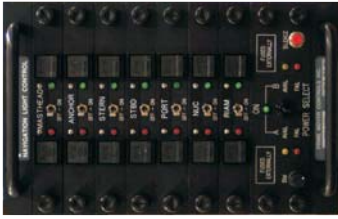
Navigation Light Control Panel
